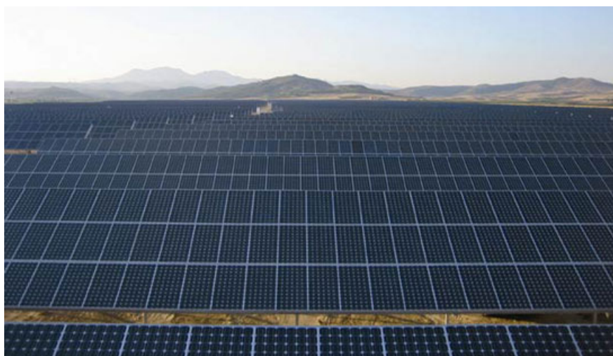
Solar energy knows no frontiers: This Vidana-based open space unit of the German aleo Solar company with its output of 4 MW is just one of many solar power stations in Spain. Source: aleo Solar.
