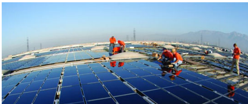
Thin-film cells for American roofs: In California, before all, solar power stations are being put up everywhere. 2-MW First Solar modules being installed on a roof in Fontana. Source: First Solar.
