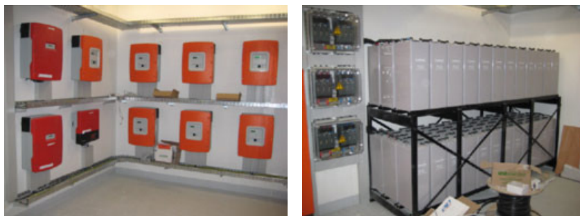
Sunny Backup: multiple inverters and a large set of batteries enable sufficient solar electric supply for a few days.
