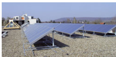
View of one of the two parts of the collector field of the solar system of the Alitherme Waldbronn. Photo: Hochschule Offenburg
