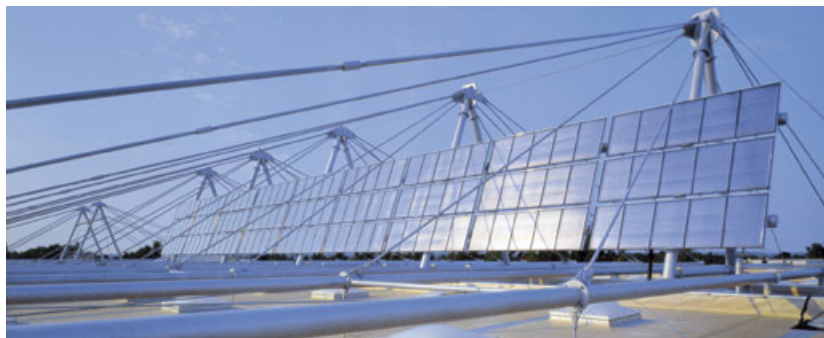
Large-scale collector of the “zero-emissions factory” Solvis GmbH in Braunschweig. Photo: Solvis; C. Richter
