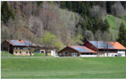
Photo: solar power system on the roof of an agricultural business in Allgäu. Source: Solarserver.de (rh)
