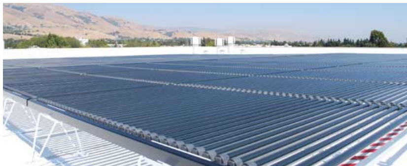
Tubular fields: Solyndra panels to cover large roofs. Source: Solyndra Inc.
