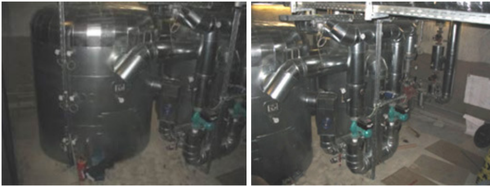
Solar storage units with a volume of 2 \times 8,5 \text{ m}^3 in the solar centre of Festo AG & Co. KG in Esslingen. Photos: Hochschule Offenburg
