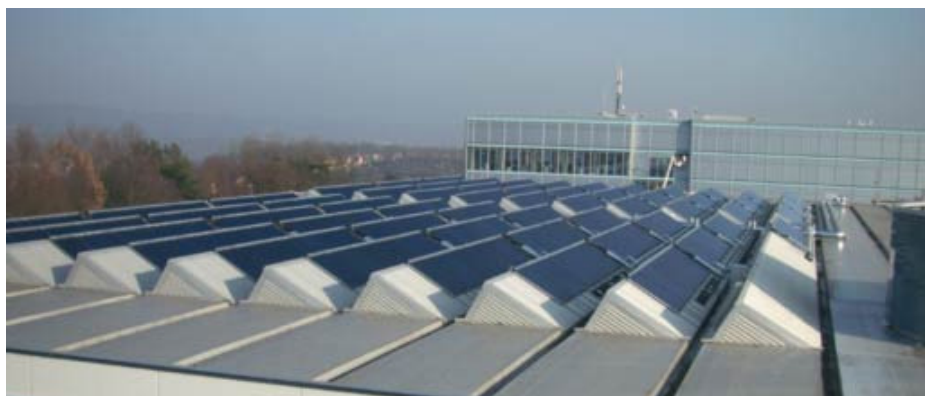
Solar heating and cooling: Field of solar collectors with a gross surface area of 1.330 m 2 on the roof of Festo AG & Co. KG in Esslingen. Photo: Paradigma Energie- und Umwelttechnik GmbH & Co. KG.
