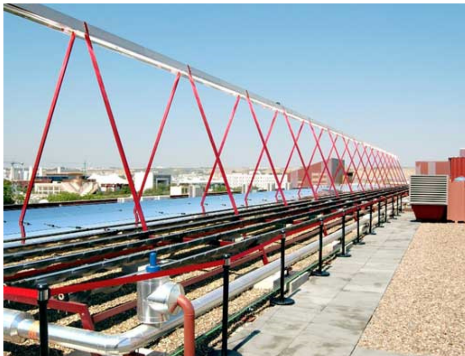
Photo: Climatisation of a building of the University of Sevilla. Chiller: Double-stage BROAD BZH 15 IX, China. Source of power: 352 m 2 linear-concentrated Fresnel collectors (Mirrox, Germany). Heat rejection: Cooling tower. Cooling: cold distribution through a central ventilation system. Photo source: Mirrox GmbH.
