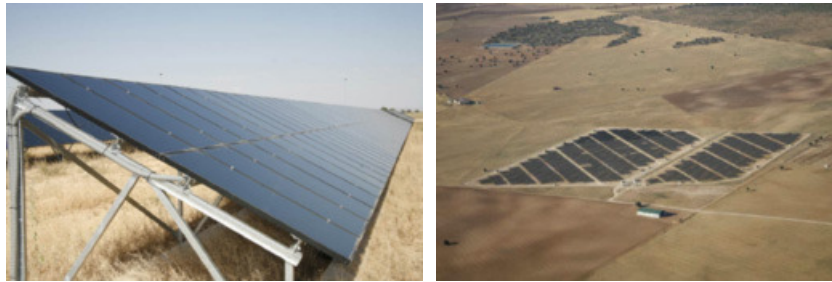
CIS modules on stands, CIS photovoltaic plant.
