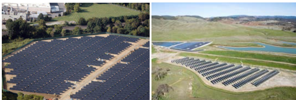
Mars Chocolate North America's PV plant at Hackettstown, New Jersey (left) and PV arrays at the LACOSAN Plant in north Lakeport, California. Courtesy: PSEG; SunPower Corporation.
