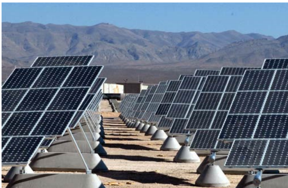
PV power plant in the US. Source: Greentech Media Research.
