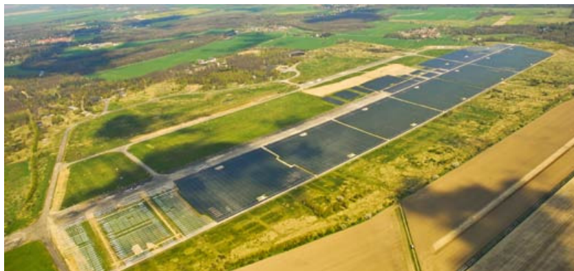
Construction progress of the "Waldpolenz" solar park at the end of May 2008.
