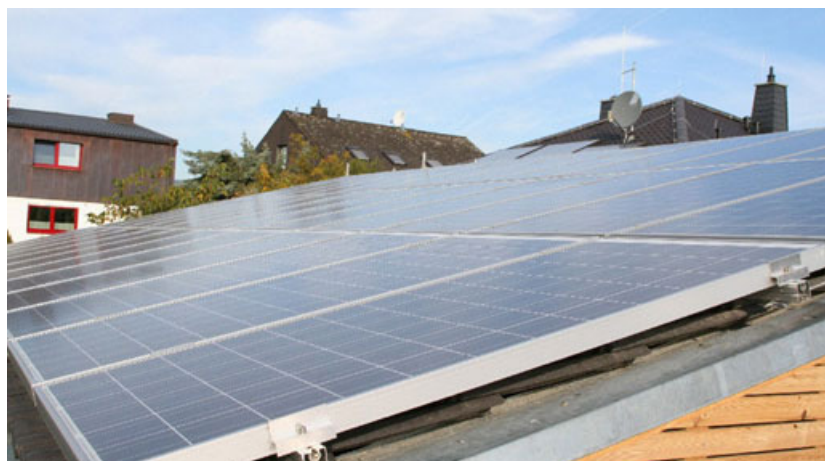
Photovoltaic system on the roof: 61 m 2 of modules; Nominal output 7,59 kWp. Source: Clemens Dahl, Architect.
