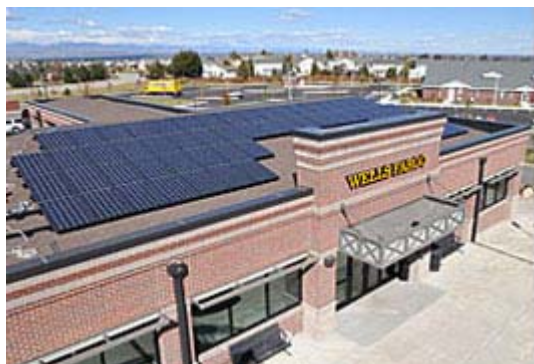
In addition to financing PV projects, Wells Fargo has installed PV systems at a number of its branches
